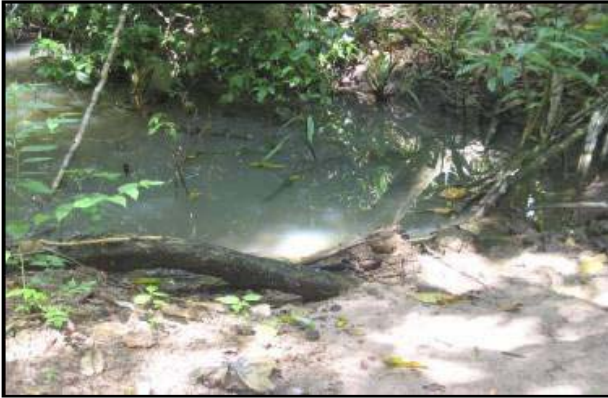
Picture 3: A faulty culvert causes water stagnation
